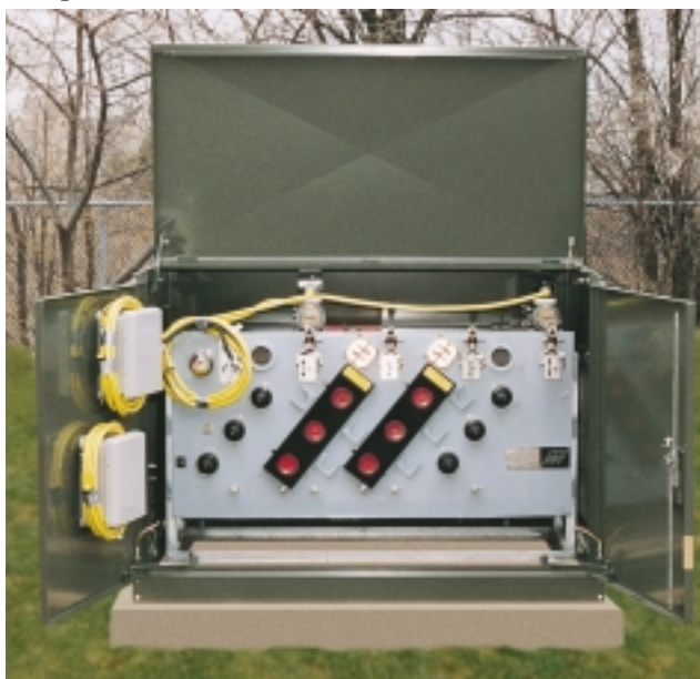
Padmount Resettable Fault Interrupter (RFI) showing two load-side ways with CT's and Controllers.
