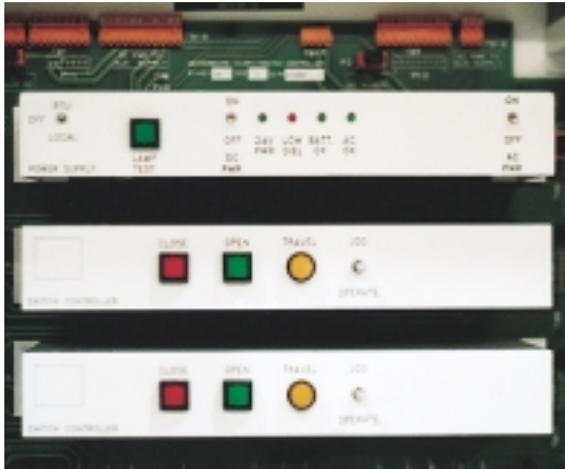
Typical Switch Controller Operator Interface
